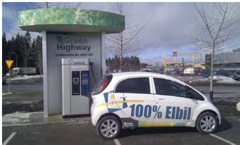
Figure 6 A canopy over rapid charging equipment in northern Sweden. Source: Vattenfall (2011)
